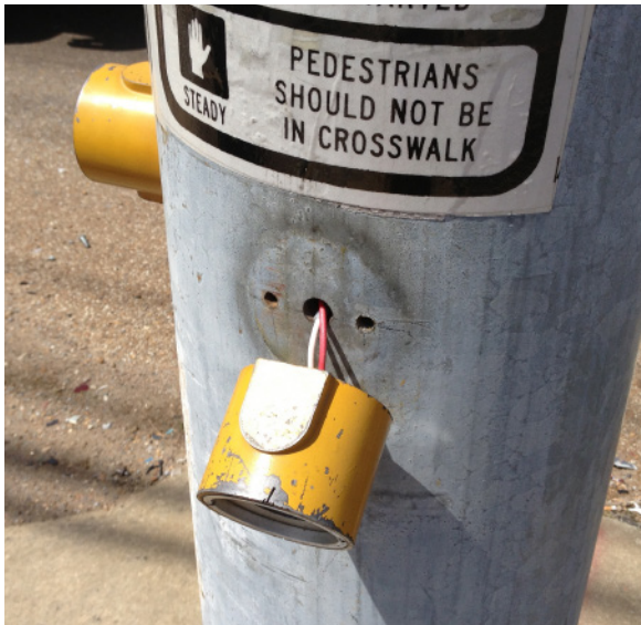
Push-buttons will require regular inspection
